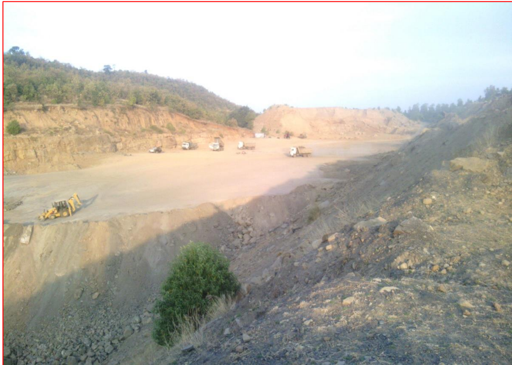
Photograph-9 Backfilling is in progress in Ghorawari oc patched in Kanhan Area
